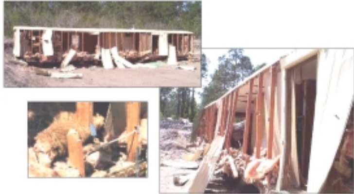
Figure 3. Damage from 12 psi Bomb Blast
